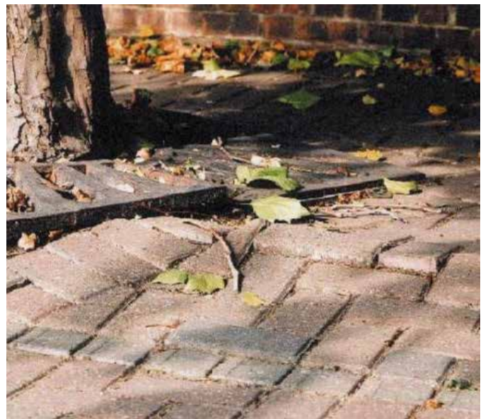
Uneven paving stones caused by unmanaged root establishment
