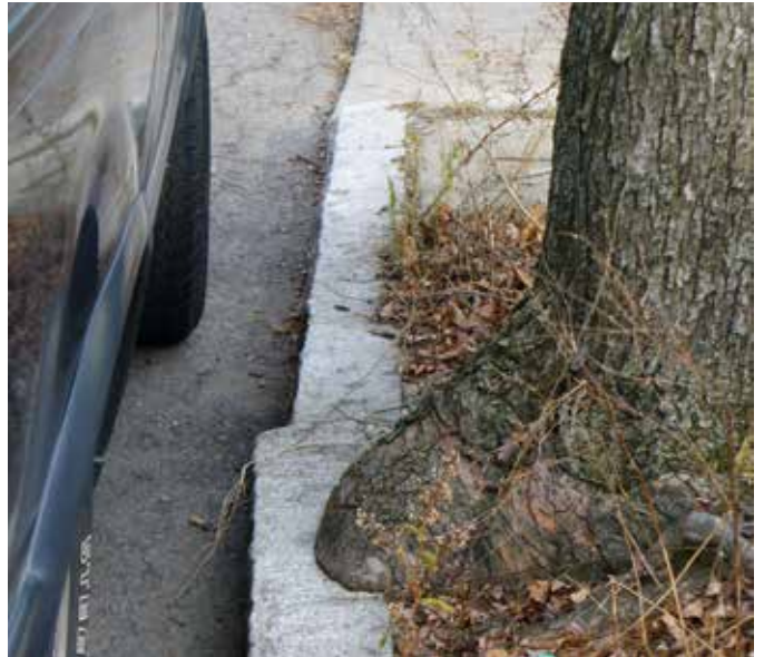
This unmanaged root system is pushing the curb out into the road, and it won't be long before this damage increases
