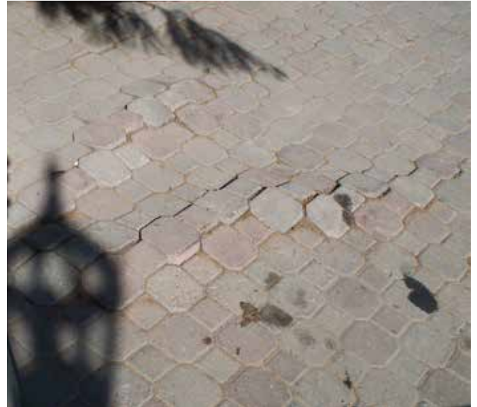
Root colonization immediately under hardscape area
