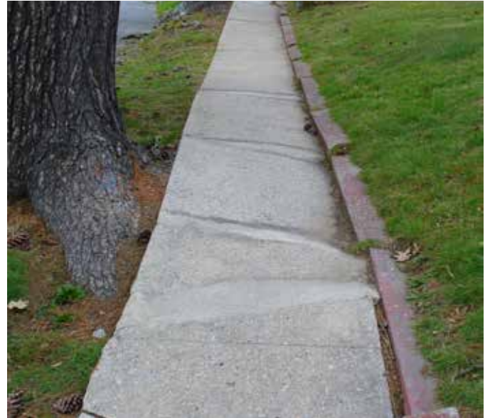
This cracking, caving, and bumpy sidewalk is typical in suburban areas where proper root management was not used in tree plantings
