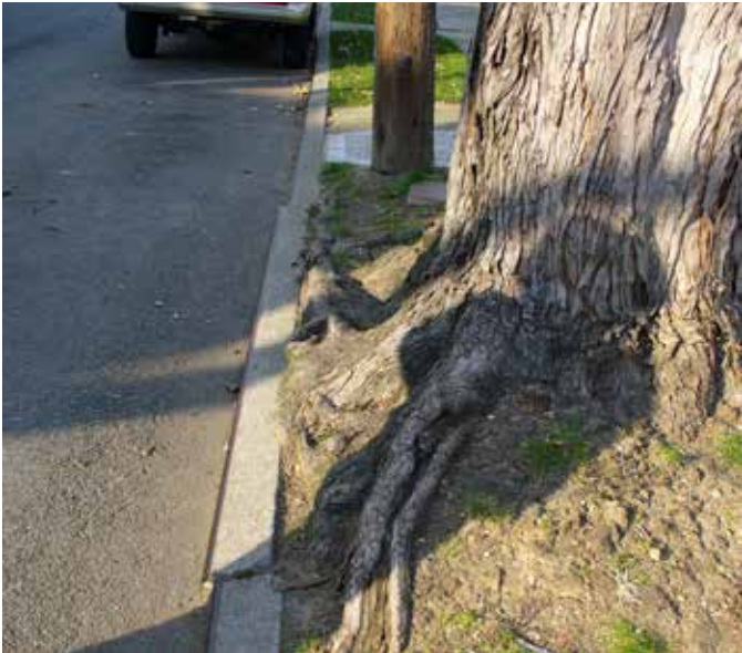
This unmanaged root system is pushing the curb out into the road, and it won't be long before this damage increases
