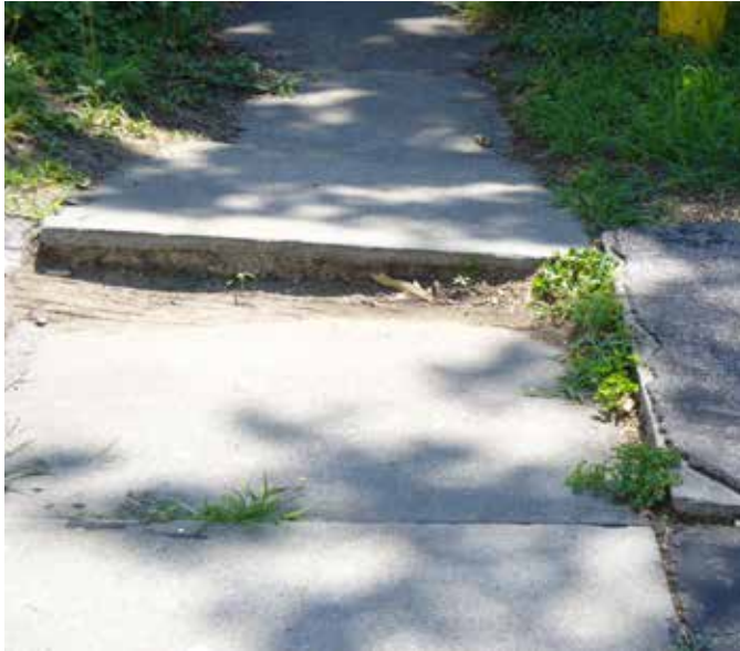
Using a RootDirector would have guided root growth to lower depths which would have prevented this upheave at the base of the tree
