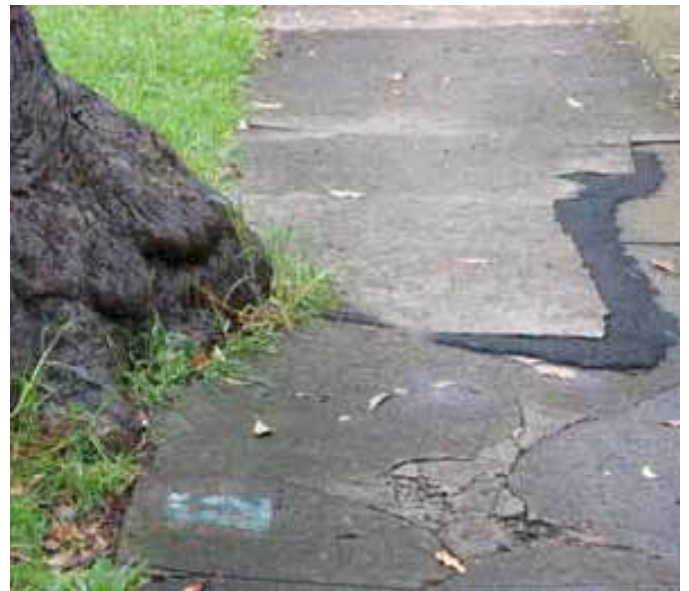
Tree roots lifting and cracking the sidewalk, a common sight in urban areas
